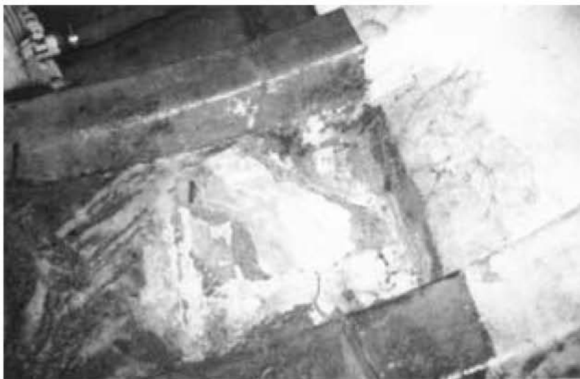
Figure 52 Hole due to grounding on anchor
